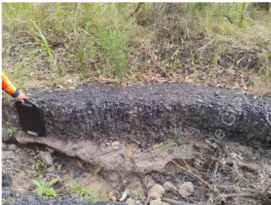
Photo 5: Abundant coal reject materials within access tracks in the far southern portion of the site (area R15) up to 0.4 m thick) (15 July 2025).
